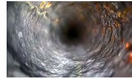
Real life problem 2 Corrosion of Piping
